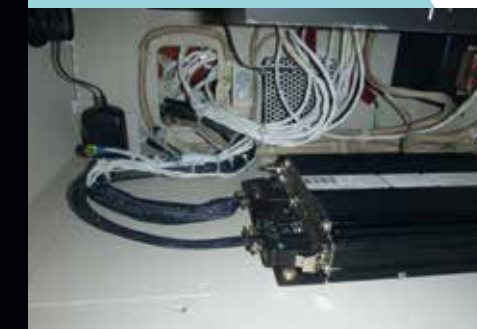
BELOW: AN ALTO DX-135 INSTALLATION ON A LEARJET 60
